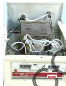
Fig: 16.20 Transformer in stabilizer
