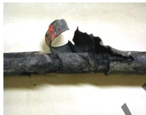
Fig: 15.23 Over heating of a cable
