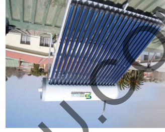
Fig (8.9) (b) Solar energy (Solar heater)
