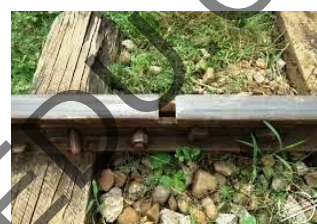
Fig (9.13) Gaps between Rail Tracks
